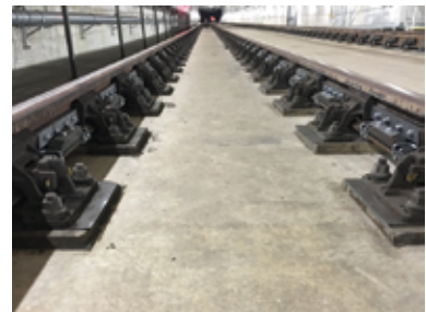
Tuned Dampers on ballastless track
