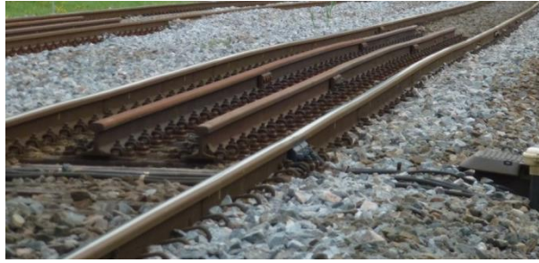
Figure 3. Transition zone with a large differential settlement.
