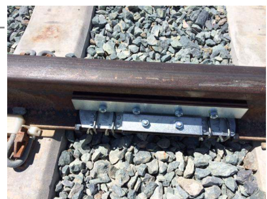
Tuned Dampers on ballast track
